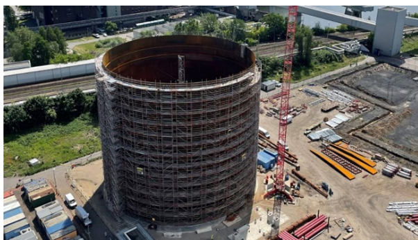
Figure 2. Germany's largest thermal storage tank is 45 m high, 43 m in diameter, and has volume of 56,000 m 3 [5].
